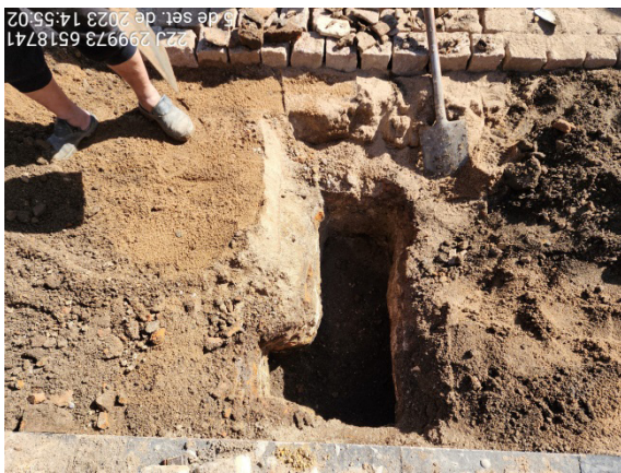
Enlargement of the test pit towards the pergola support beam (white arrow), and attempted expansion parallel to the beam (red arrow). Iha)
