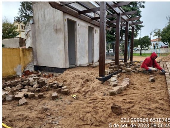
Status of the patio area recorded in September 2023. Pergola and beam added to the structure bathroom area, layer of sand embankment 20cm and laying cobblestones
